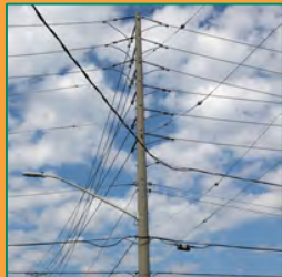
680.7 km Overhead Circuitry
